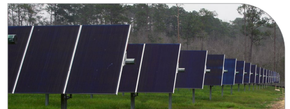
Wing Solar Farm | Wing, AL 🖱️
